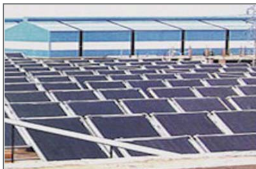
Fig 3.17: Solar Panels to trap solar energy
